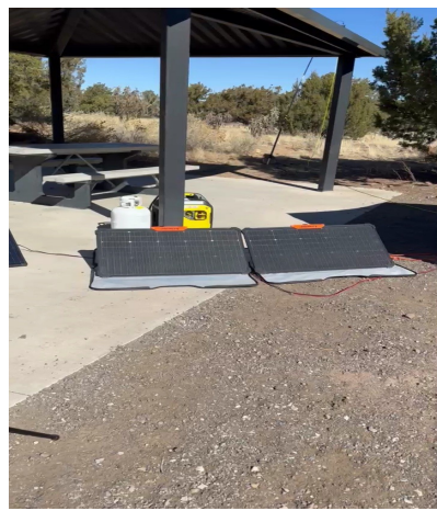
Solar System & Backup Genera-
